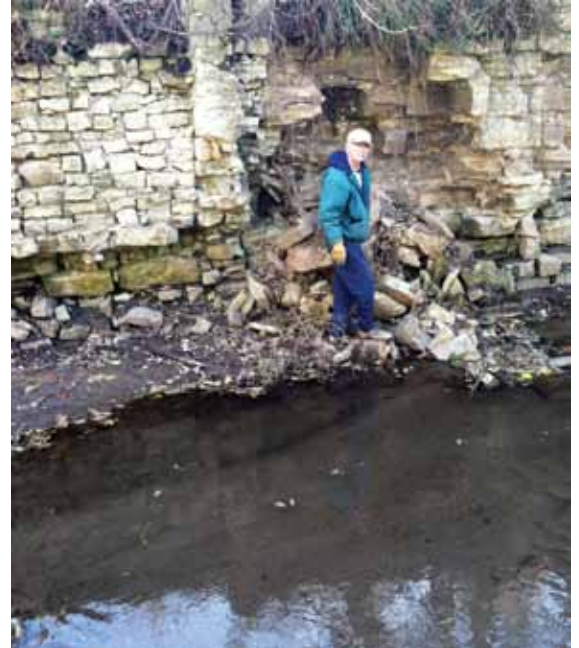
Volunteer Russ Mayer in front of mill ruins eroding from creek bank.
