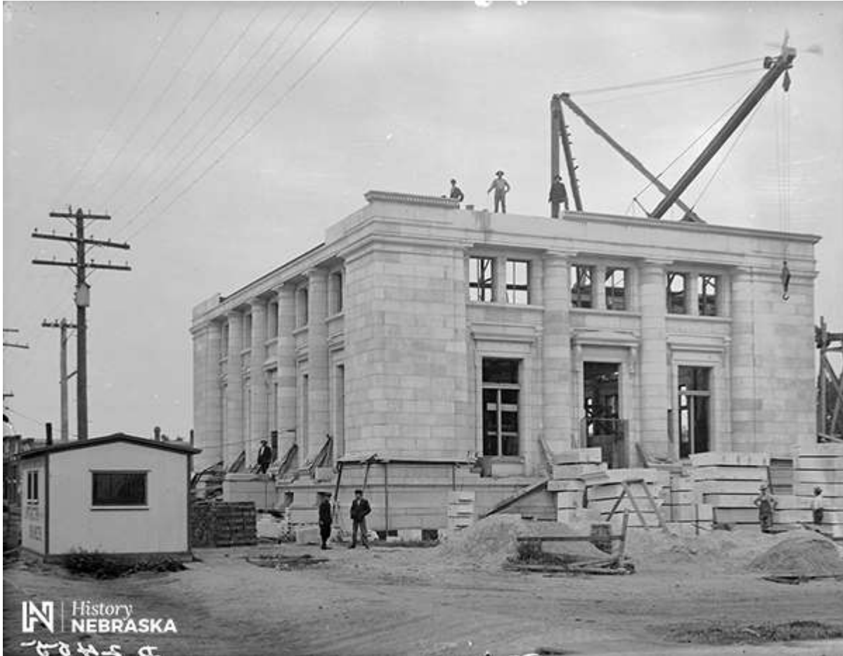
Photo: Kearney Post Office under construction in 1907. Today the building is home to the Museum of Nebraska Art and is listed on the National Register of Historic Places. Photo by Solomon D. Butcher. History Nebraska RG2608-0-2455
