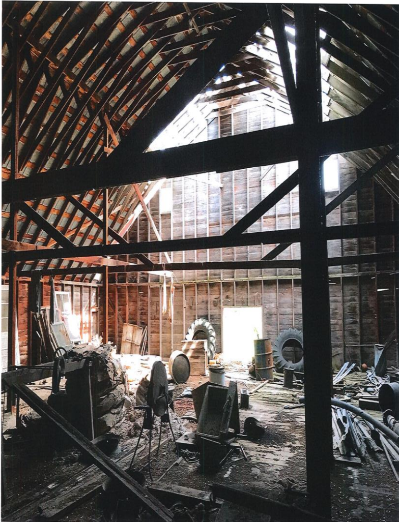
Hayloft picture taken from North to South. Can see tin missing on south (east & west).
